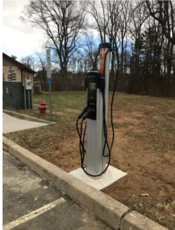
Image 18. Electric Vehicle Charging Station, located at the Department of Public Works in Middletown, PA.
